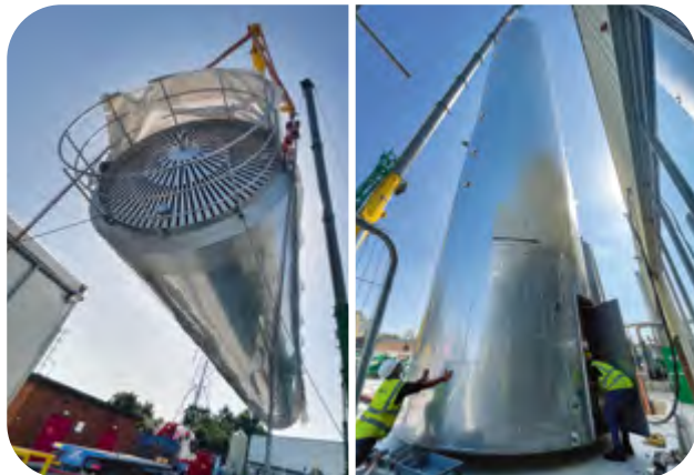
Thermal store installation taking place at our Beckton site, part of the new heat recovery system to improve energy efficiency and cut carbon emissions.
